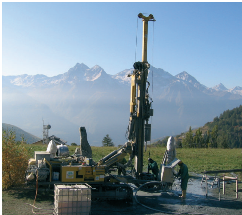
Installation of a borehole heat exchanger in the Aosta Valley, Italy. Copyright: GRETA project. ■
